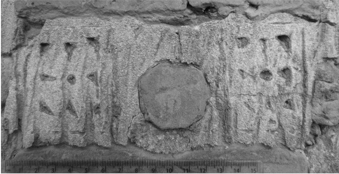
Fig. 22 – Geometric mortar incisions on the portal exterior of the Mengücek Ghazi tomb © R. McClary
