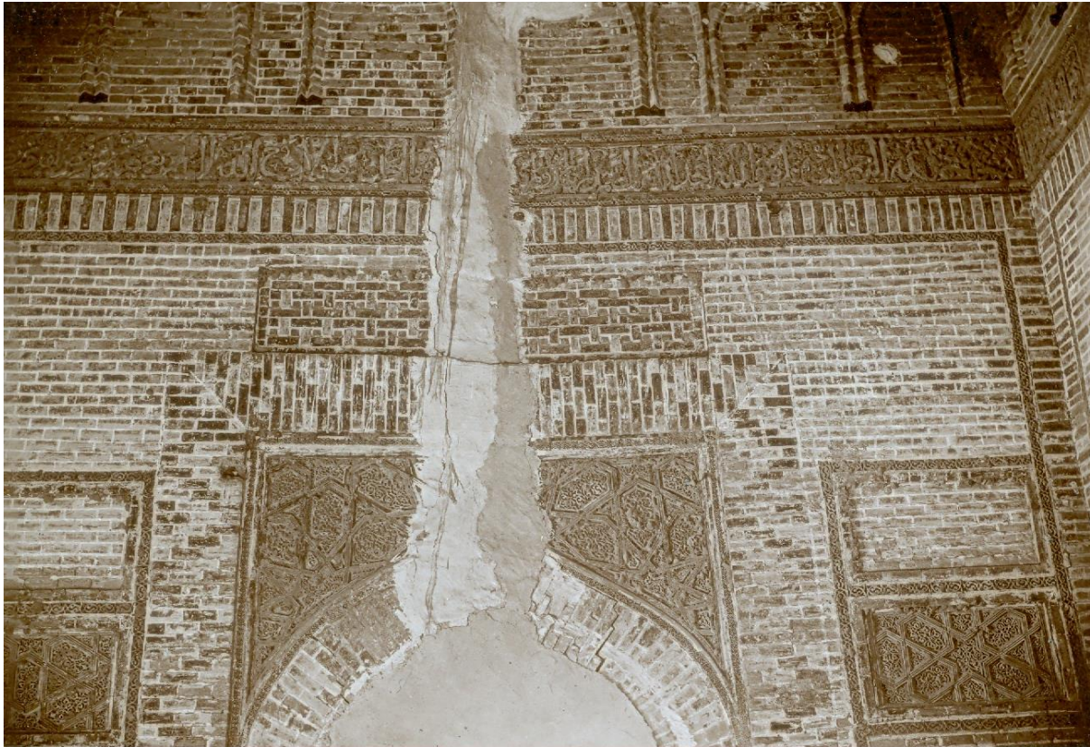
Figure 22 Southeast interior wall of the mashhad , photograph by F. Sarre © Max van Berchem Foundation, Geneva
