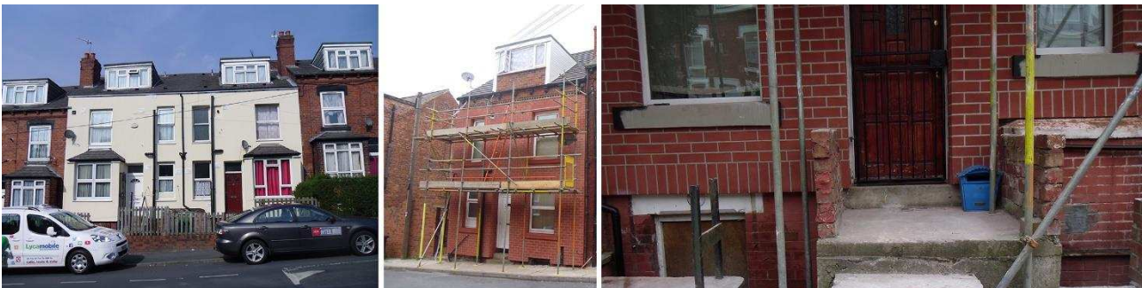
Figure 12. Typical examples of non-permeable external wall insulation in Harehills. The character of the houses has been compromised whichever of the two approaches is used – to the left is a render finish which makes no attempt to respect the detailing beneath, and to the centre and right, a finish which replicates the appearance of the bricks and lintels. Since the finish stands forward of the frieze, it diminishes its prominence, and poor detailing could lead to thermal bridges and internal dampness. ©Joanne Harrison.
