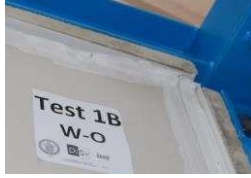
7. Rupture of panel portions
