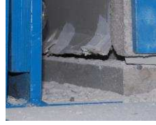
5. Corner crushing of panels
