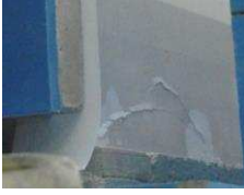
4. Crack in panel
