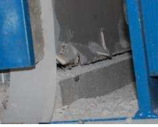
6. Collapse of panel-to-frame fixings
