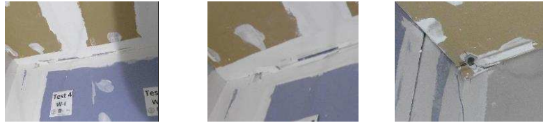
3. Detachment between walls and structural elements 6. Collapse of panel-to-frame fixings 7. Rupture of panel portions
