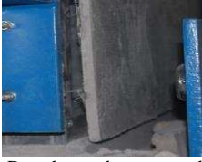
3. Detachment between walls and structural elements
