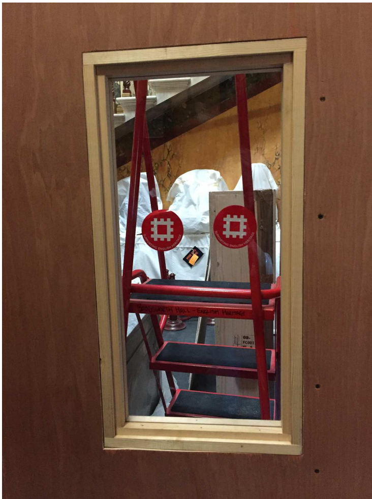
Figure 10: Observational windows in the protective hoardings were opened up in the entrance hall later in the first season to give visitors a sense of what was being protected behind them.
