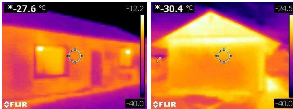
537 538 Figure 17. Thermal image of south wall (left) and west gable end wall (right).
