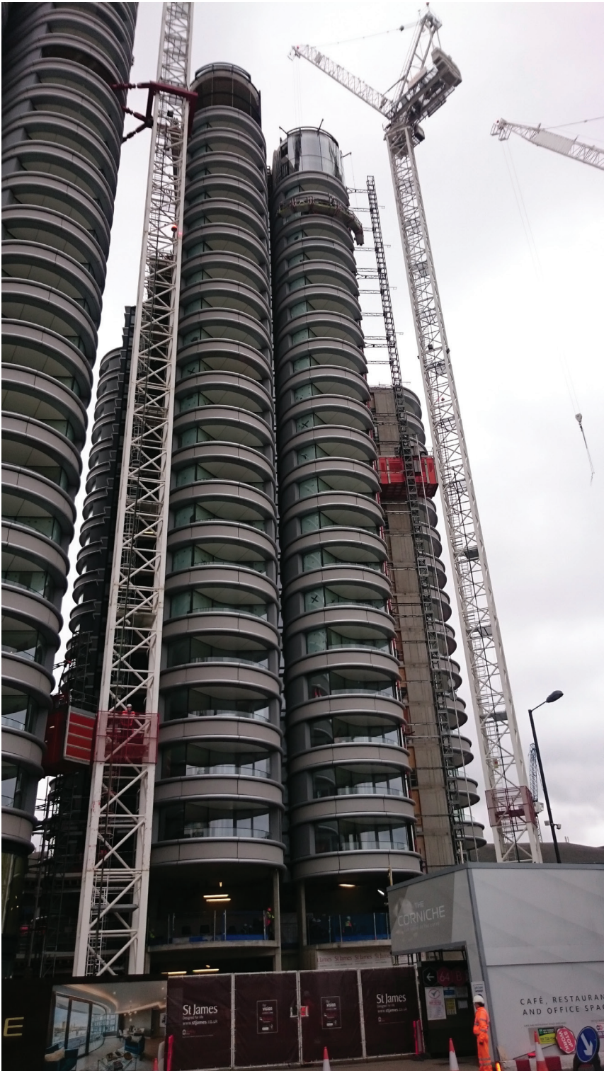
FIGURE 2 Luxury apartments on the Thames under construction (photo by the author, March 2017)
