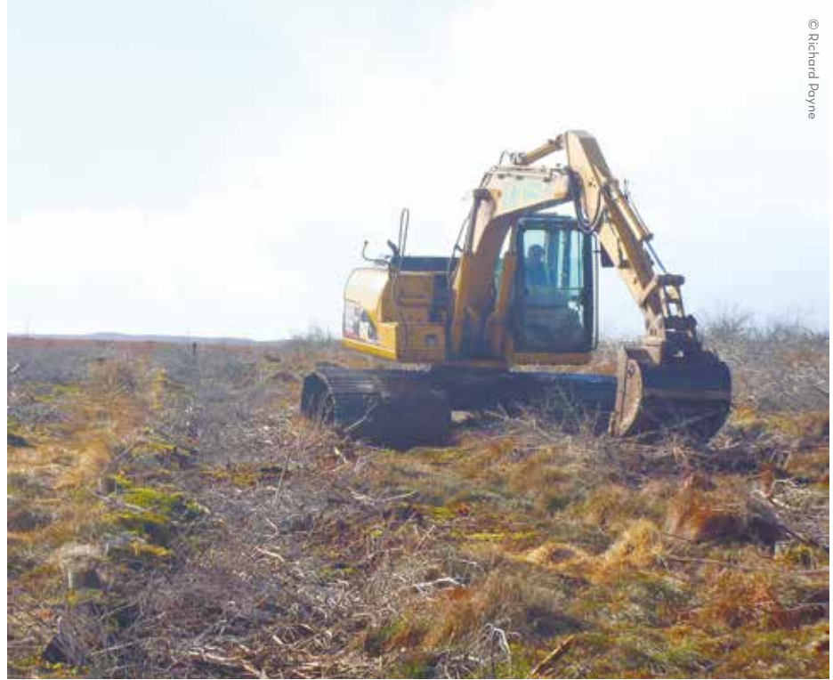
Figure 4: Forest-to-bog peatland restoration underway at RSPB Forsinard. In this 2014 image the digger is conducting secondary treatment, compacting previously felled-to-waste trees into the plough furrows.
