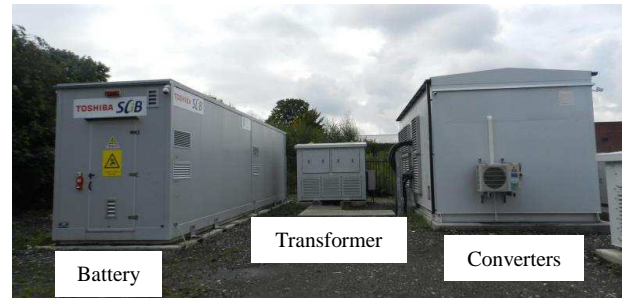
Fig. 10. (a) Block diagram and (b) photo of the 1 MWh/2MW WESS plant.
