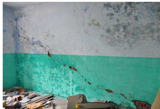
(b) Large crack on wall piece
