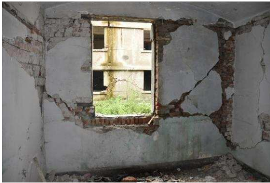
(c) Severe cracks on wall piece
