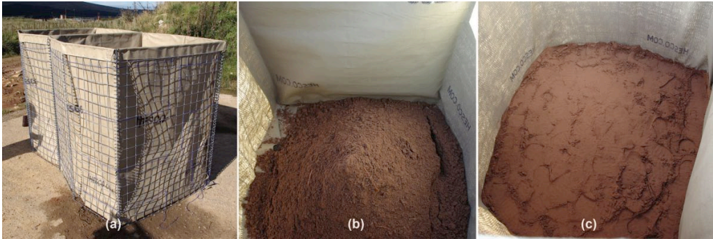
Figure 3. Gabion filling method: (a) deployment, (b) addition of fill material layer and (c) distribution and compaction of layer.
