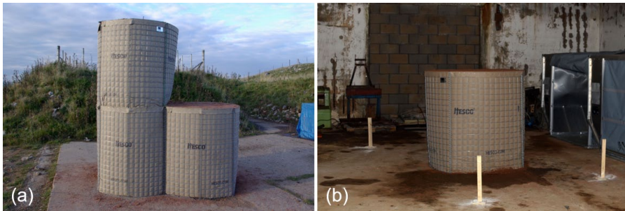
Figure 4. Gabions after filling (a) exterior gabions PI-P3 and (b) interior gabion I1.
