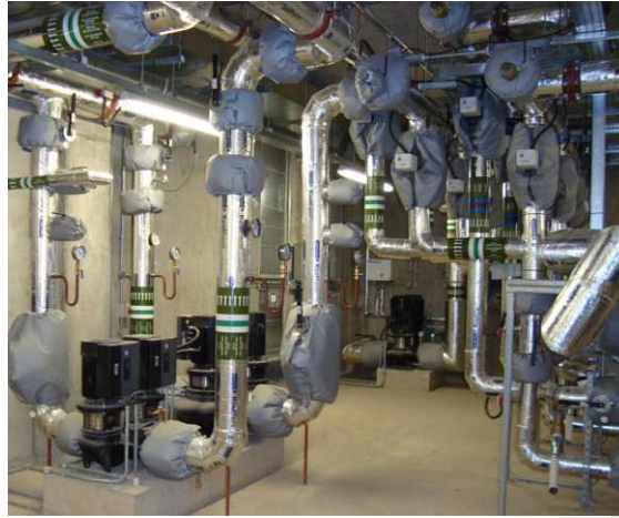
Figure 6: The system circulating pumps installation. Heating and chilled water header circuit pumps are in the foreground and the ground loop pumps in the background.
