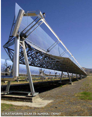
Fig. 1: ACUREX distributed solar collector field.
