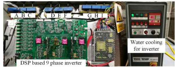
Fig. 4. DSP based 9-phase inverter.
