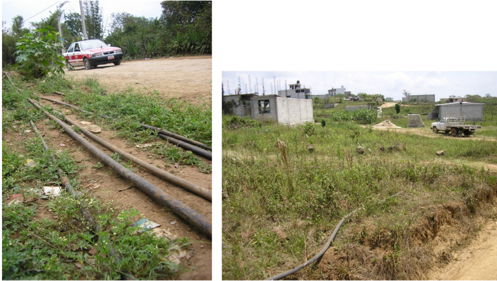
Fig. 11. Pipes on access road/entering Loma Bonita. Source: Mauro Castro (2007), Melanie Lombard (2007).
