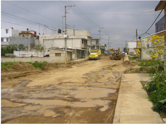
Fig. 19. Start of works to pave the main street, Moctezuma. Source: Melanie Lombard (2007).
