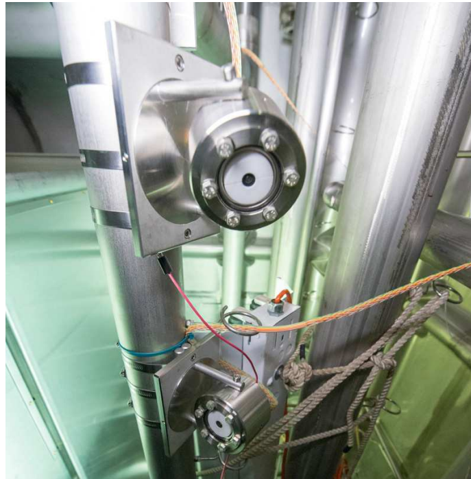
Figure 11. Two camera modules and mounts clamped to 3" SCH cryogenic pipes in the 35t cryostat.
