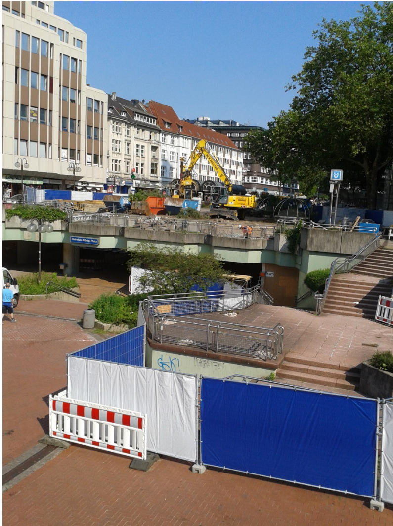
Figure 2: Picture of Heinrich-König-Platz being redeveloped in July 2013. Hans-Sachs-Haus is in the background (partly obscured by the tree)
