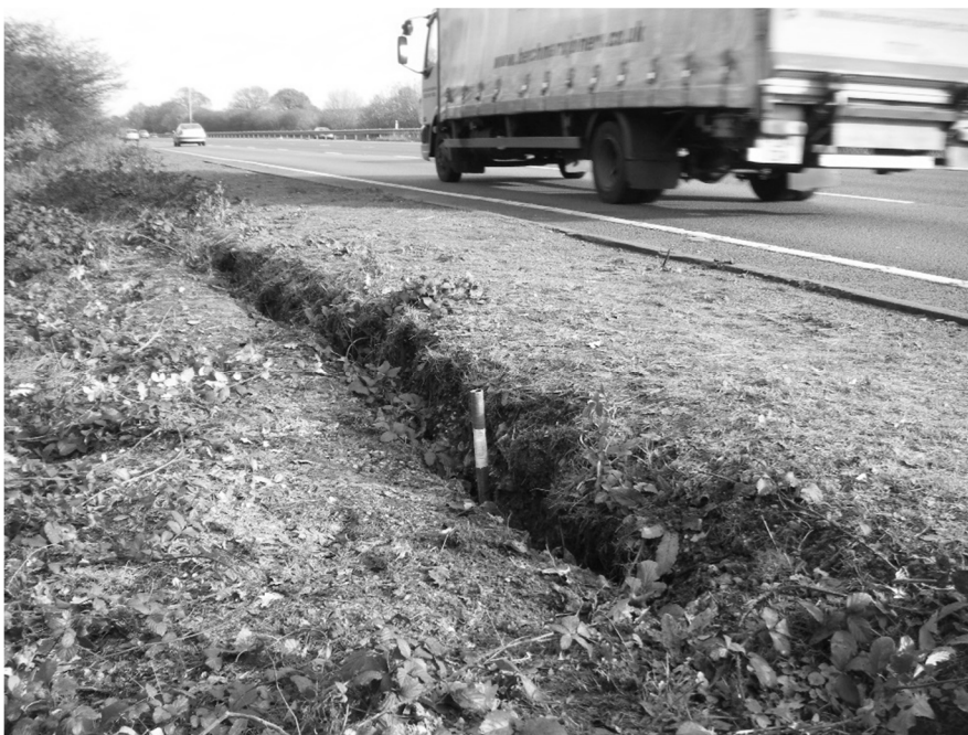
Figure 4b: Tension crack at the crest of a highway embankment slope (photo courtesy of David Patterson, Highways England)
