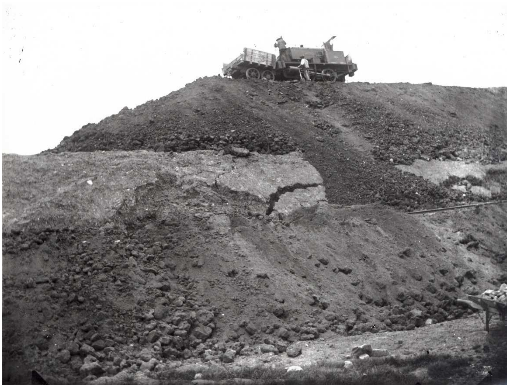
Figure 2: End tipping of a Great Central Railway embankment in Whetstone around 1897 (Photo reproduced with permission of The Record Office for Leicestershire, Leicester and Rutland, on behalf of S.W.A. Newton)
