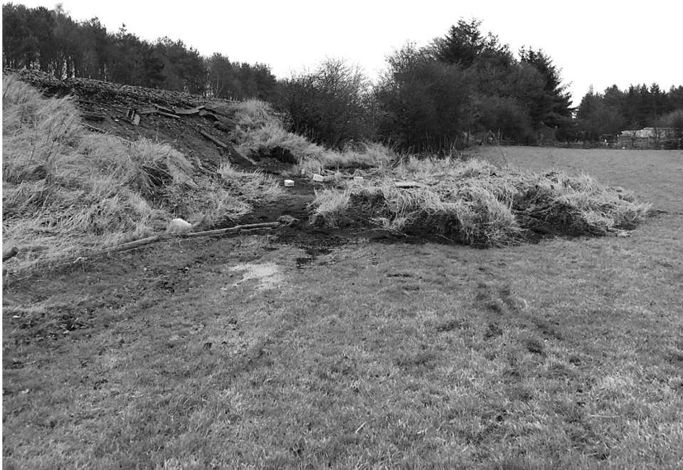
Figure 5b: Shallow failure of a railway embankment slope at Willow Gap on the Newcastle to Carlisle railway line (photo courtesy of David Hutchinson, Network Rail)
