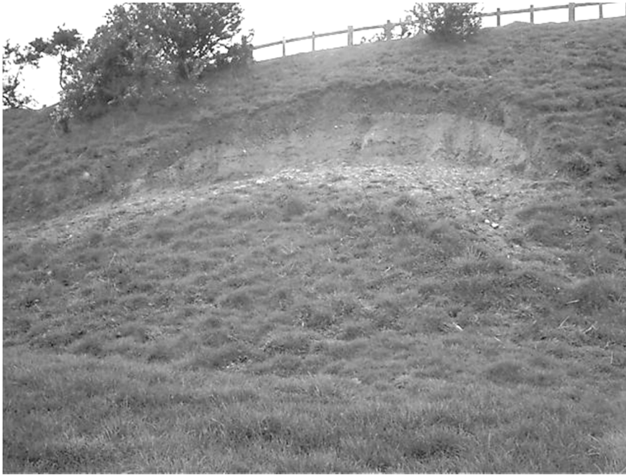
Figure 4a: Failure of a highway embankment slope. The compacted fill and topsoil are clearly shown (photo courtesy of David Patterson, Highways England)
