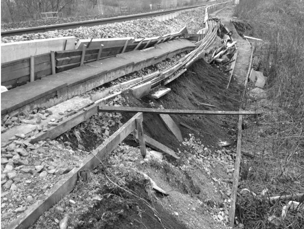
Figure 5a: Failure of a railway embankment slope at Leighton Buzzard (photo courtesy of Tony Butler, Network Rail)
