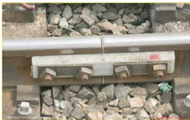
Fig. 1. Insulated Rail Joints (IRJs) [6].
