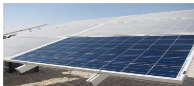
Figure 1. PV system after one month of soiling at the Qatari QEERI Solar Test Facility [4].
