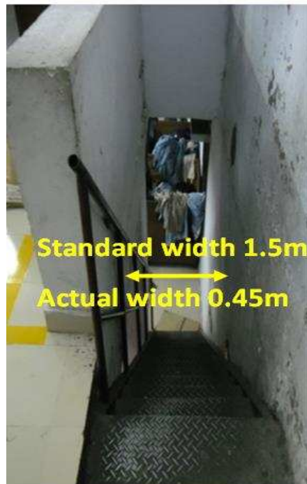
Figure-1: Hard factors: Stairway does not meet regulation.
