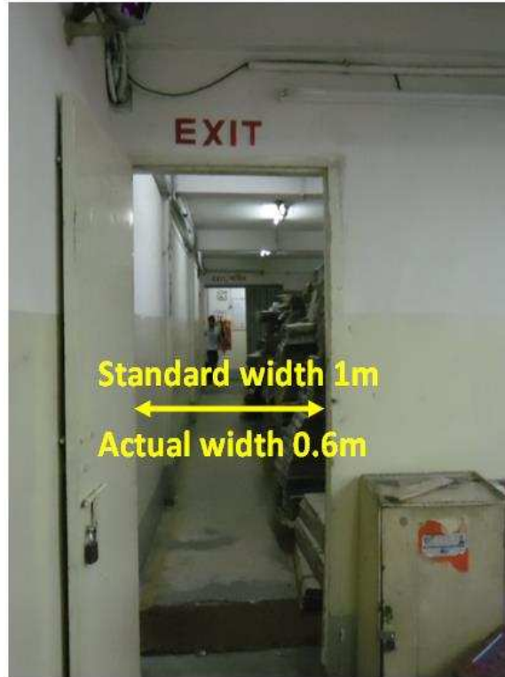
Figure-2: Hard factors: Exit door does not meet regulations.
