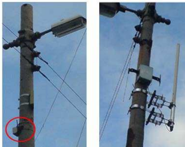
Fig. 14: Wireless link enhancement methods; (a) Adding relay point, (b) Using high gain antenna on the data gatherer
