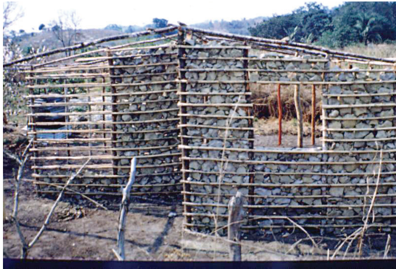
A typical traditionally-built house showing how cracks in walls can provide ideal habitats for the triatomine bugs that transmit the parasites which cause Chagas disease, 2002. WHO/TDR
