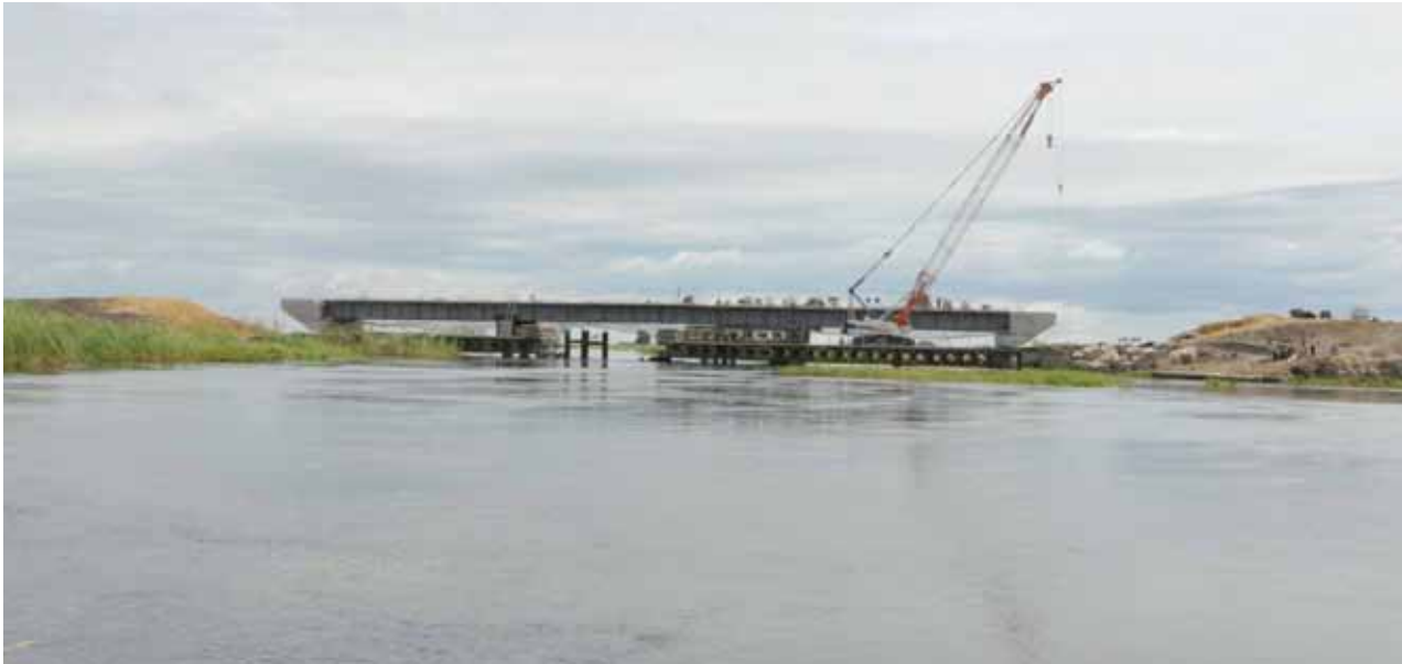
Figure 3: Reconstruction of the bridge on the Mongu-Kalabo Road near Mongu Harbour. The road, linking the districts of Mongu and Kalabo in western Zambia, was extensively damaged during a higher than normal flood event in 2003/2004 season. The road is envisaged to be a gateway between Zambia and Angola for enhanced economic interaction between the two countries. Though the road and bridges are being constructed there is no information on the impact the construction of this road infrastructure will have on flood extent regimes, river channels, silt deposition, or on fish and wildlife movements. This makes it more significant to have in place a flood pattern monitoring system that will facilitate for disaster management preparedness as well as biodiversity monitoring in the wetland (Photograph: Helmschrot, 2015)
