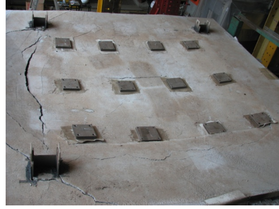
b) Failure mode
