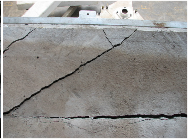
b) Fracture of reinforcement
