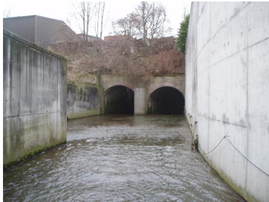
Culvert on Bradford Beck, enabling levelling of land and development to take place
