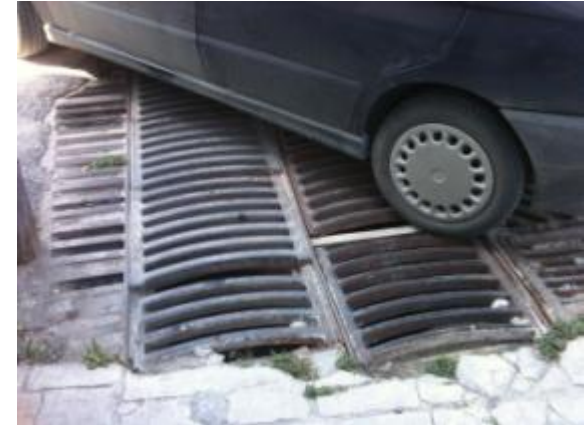
Gully grate in Kassandria, Halkadiki, Greece
