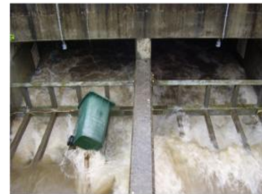
Inlet screen at large culvert under pressure
