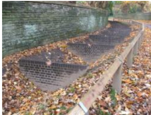
Stepped swale in Mayfield Road, Bradford
