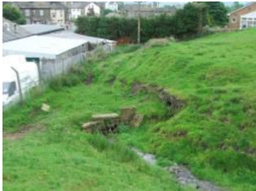
Makeshift screen at culvert entrance
