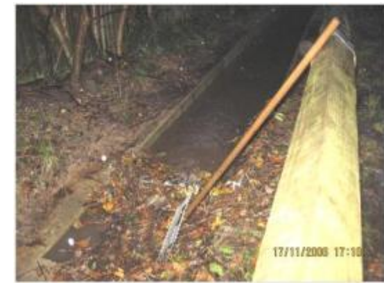
High water levels due to blockage of culvert inlet
