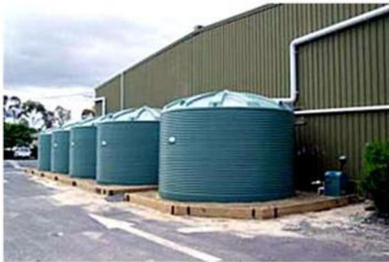
Industrial application of rainwater tanks at Hume depot, Australia (Tony Weber)
