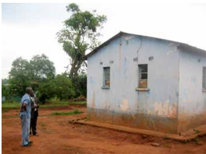
House with crack allegedly from mine blasting
