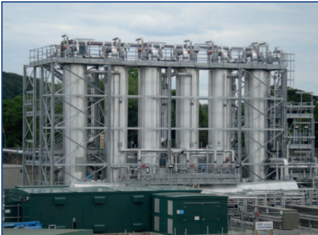
The BioThelys thermal hydrolysis plant at Esholt is designed to treat a nominal throughput of 30,000 tonnes of dry solids per year of a mixture of primary and secondary sludges which are produced both at the Esholt works itself as well as sludge imported from other sites. A BioThelys plant at Oxford is in construction phase with a process commissioning planned for the beginning of 2014.
