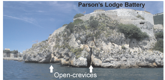
Fig. 4.- Rosia Bay site (R in Fig. 1B) and its Parson's Lodge southern flank. Extensional open-crevices partially filled by tsunami sediments.
