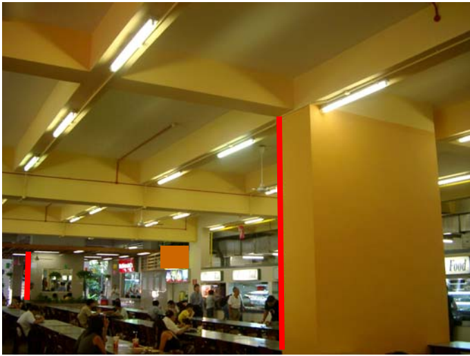
Figure 8a - Singapore Polytechnic floor viewed from below, with near and far columns highlighted
