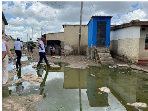
Flooded road and raised toilet (before rainstorm)
