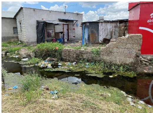
Full drain with rubbish (before rainstorm)
