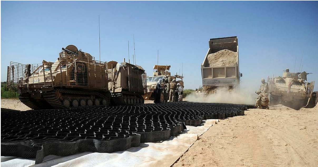
Figure 3. Royal Engineers and Afghan civilian contractors building route Trident using Neology (Source: MOD, UK MOD Crown Copyright, 2010)
