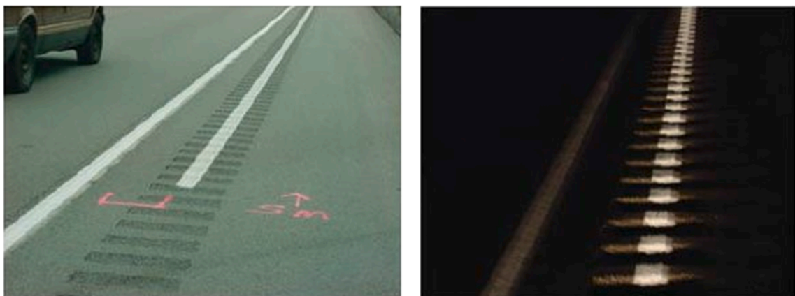
Figure 6. Night-time visibility of line marking within the rumble strip, taken from (FHWA, 2015).
