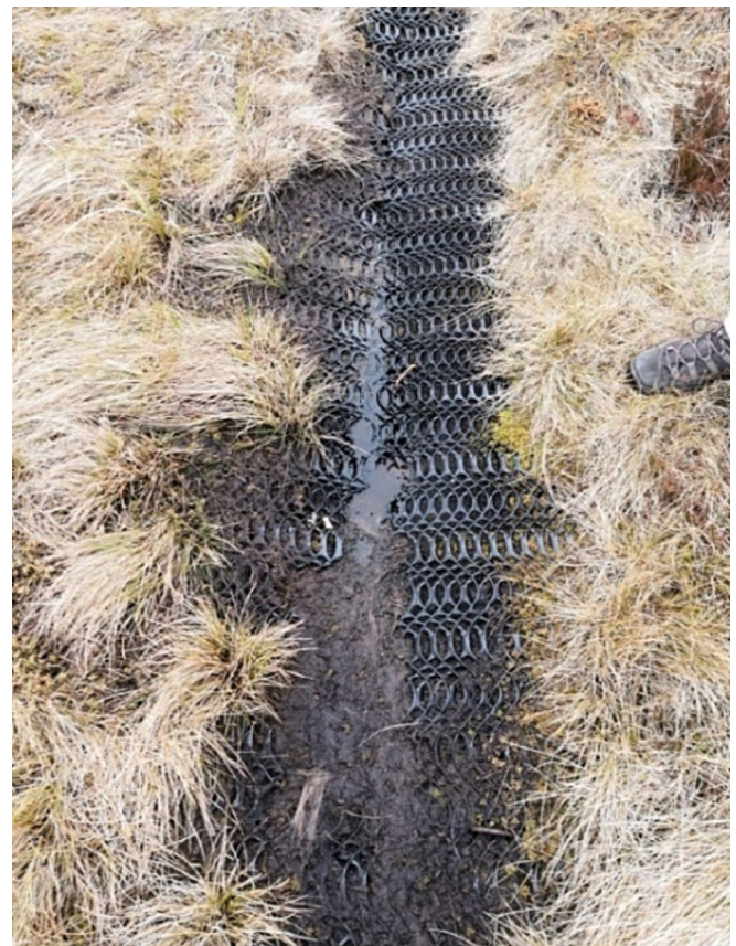
FIGURE 5 Area of failed track in a rutted section.
