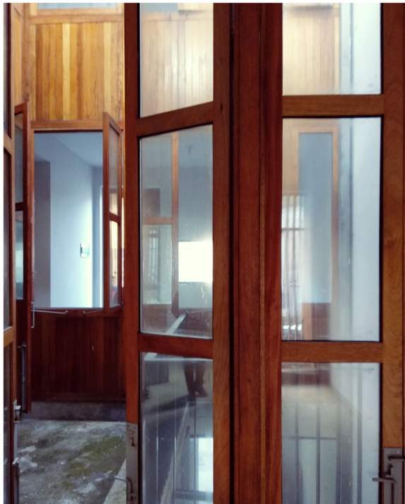
Fig. 11 The courtyard is covered with moss, partly due to a lack of protection from humidity in the design of the enclosed wooden shutters (Source: the author)
