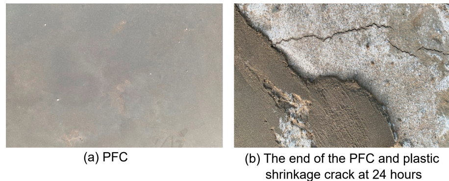
Figure 8. Concrete surface finish after the power floating of in situ large-scale slabs: (a) inner area, and (b) edge of slab.
