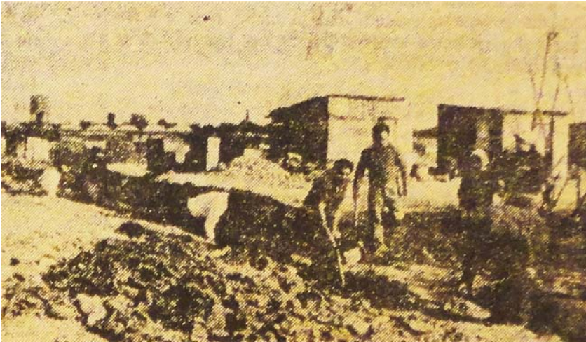
Figure 1. Residents of Villa Rotonda Varela opening trenches for fresh water pipework. Source: La voz de las villas , February 1965.
