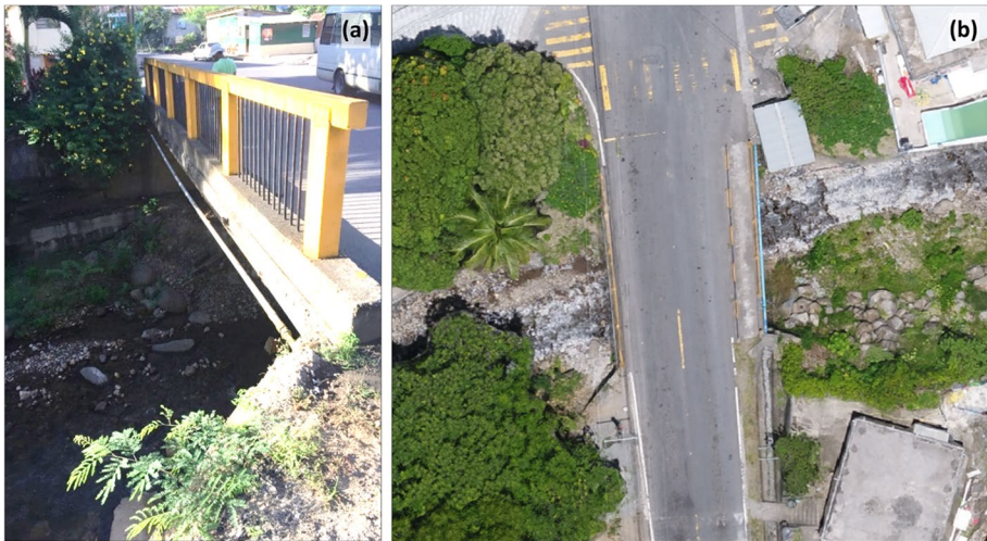
Fig. 6 Example of the smaller bridges, Colihaut main bridge (a) from left bank downstream, and (b) from drone orthophoto
