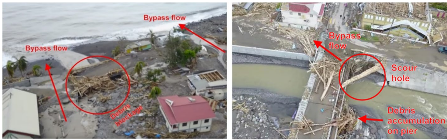
Fig. 10 Post Maria damage in (left) Coulibistrie Reach showing bypass flows and debris build up, (right) Local bridge scour exacerbated by debris at Roseau Bridge 3
