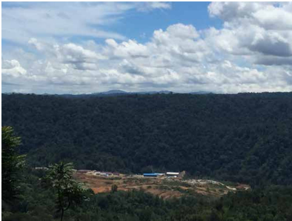
The PT North Sumatra Hydro Energy is clearing the project site (FoE US2019)
