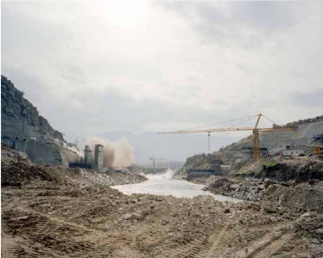
Explosion at Deraluk Reshawa dam construction site, Deraluk, Amadiya district, Iraq. 21 november 2018. (c) Alex Kemman
