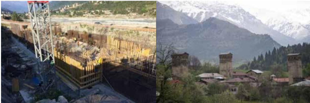
Left: Construction of Mestiachala HPP in 2017. Ancient Swan towers in Mestia seen on the backdrop at the foot of the mountain. (Photo by Austrian construction company Convex 10 ). Right: Ancient towers of Mestia in their natural landscape (CEEBWN 2018).
