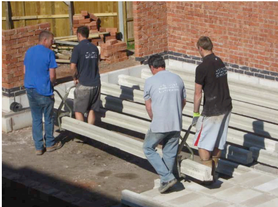
Photo 4.2: Non-compliant PPE but fairly good ergonomics and OSH practice on the aspects that the workers considered important (Photo Gibb).
