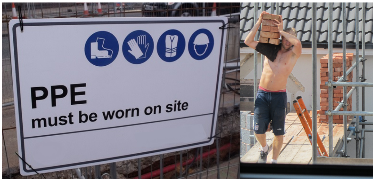
Photo 4.1: PPE sign by site entrance ignored by micro construction workers (Photo Gibb)
