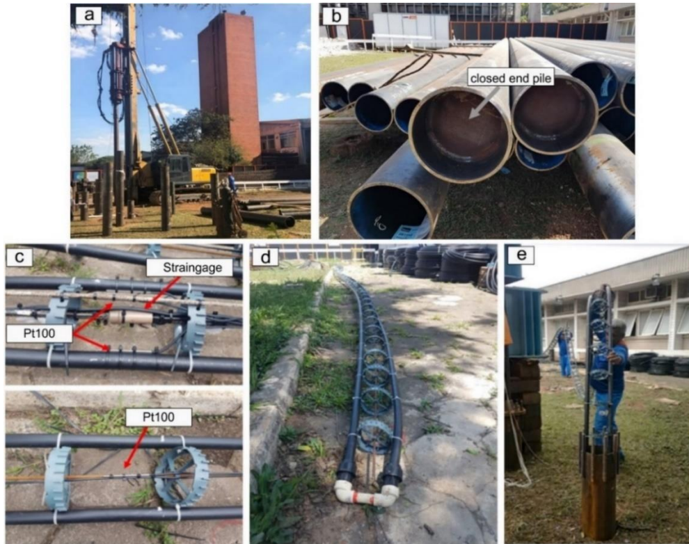
Figure 1. Installation of the test energy piles: (a) pile installation; (b) closed end test pile; (c) pile instrumentation; (d) single U-tube; (e) installation of U-shaped pipes into the pile foundation.
