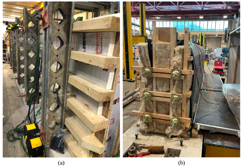
FIGURE 5 Formwork used at (a) ICL and (b) UoL. ICL, Imperial College London; UoL, University of Leeds
