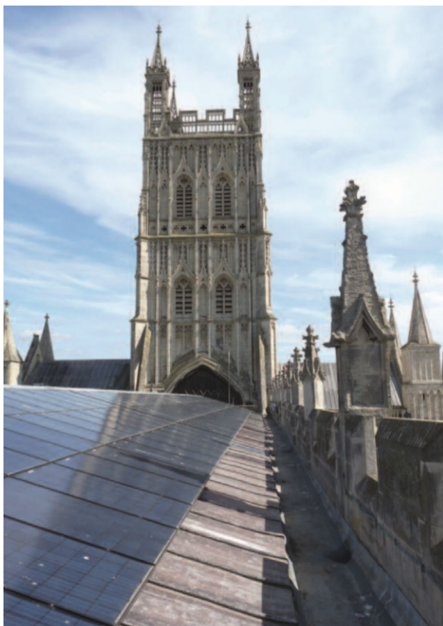
FIGURE 1 A view of Gloucester Cathedral roof upon completion. Image provided by Mypower Solar 15
