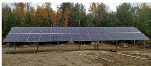
Fig. 12 Examined PV modules placed outdoor after the PID test is completed. The PV system consists of 28 modules distributed among two strings, each string comprising 14 modules.
