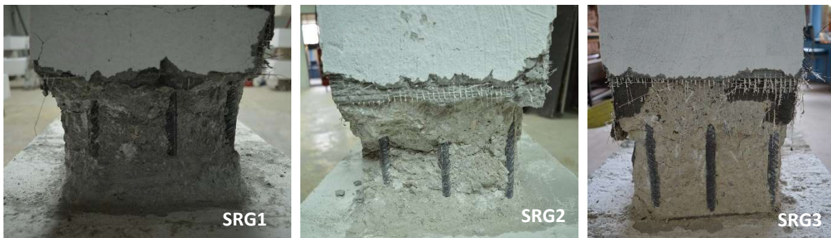
Fig. 15: State of the core cross section in the critical region after removal of the textile.
