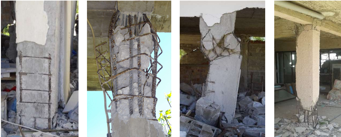
Fig. 1. Damage in RC columns due to old-type detailing (photos are taken by the authors).
