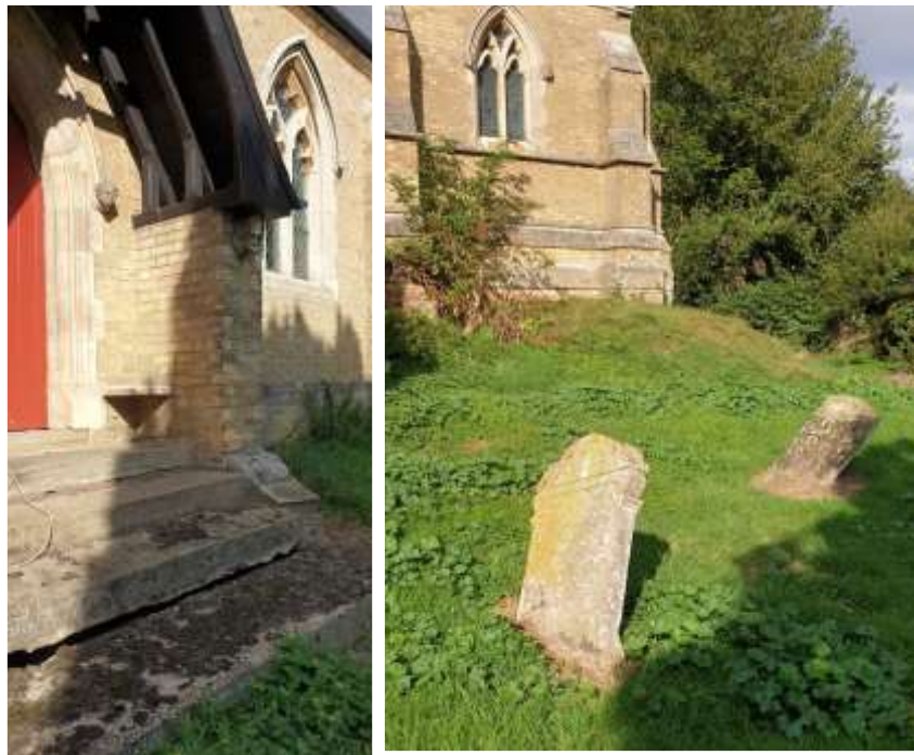
Figure 10: Subsiding steps at the Church entrance and collapsing gravestones in the churchyard at Ramsey St Mary's, Cambridgeshire. Built in 1859, the church was constructed on peat and soft clay using a foundation of wooden piles. It has remained relatively stable, although the spire had to be removed in 1920. By contrast, the surrounding land has subsided by several metres, leading to damage to churchyard monuments and necessitating the demolition of the Vicarage.
