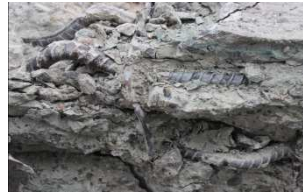
(f) Re-bar buckling (TRC-0.6-0)
