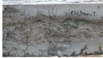
(c) Concrete cracks in tension zone (TRC-0.5-25)
