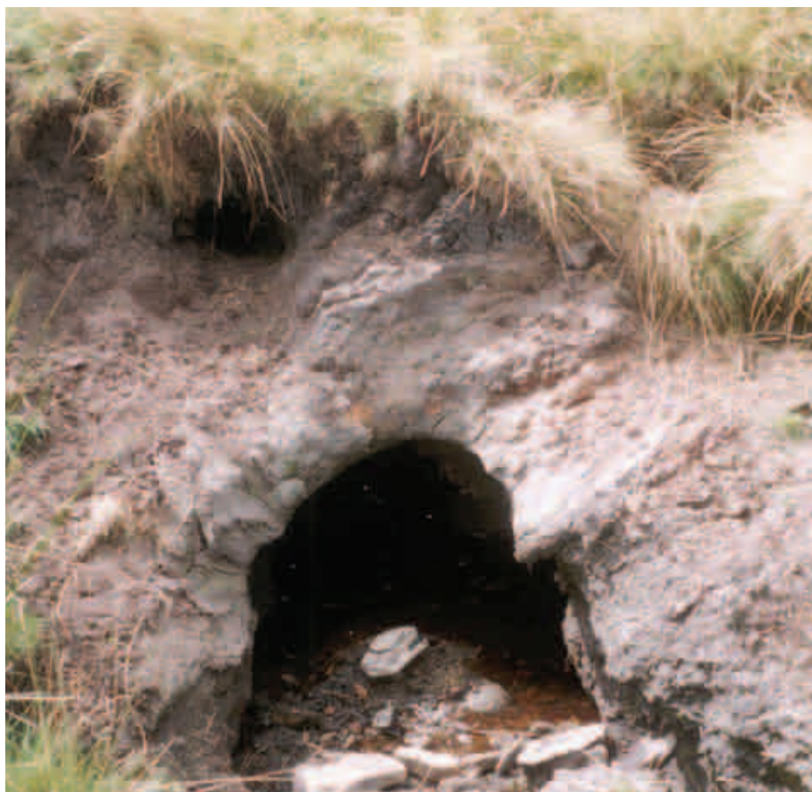
Figure 1. A soil pipe outlet with coarse sediment delivered from its base.
