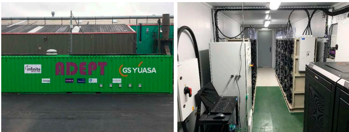
Figure 6. Battery storage cabinet of the ADEPT system (physical part).
