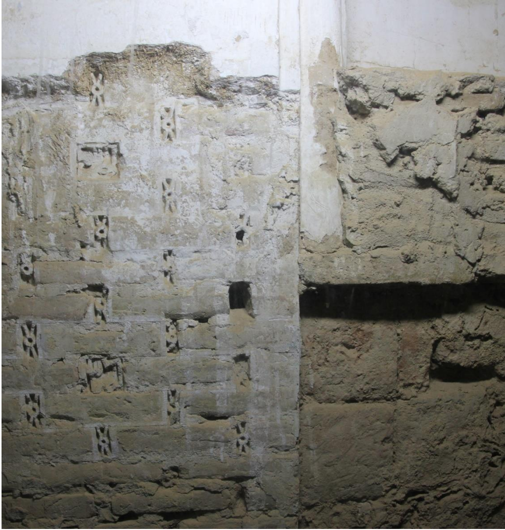
Figure 7: construction break beside the blind recess to the right of the mihrab, with the later engaged column extending down behind the (lost) lustre inscription band to the height of the top of the star and cross tile dado
